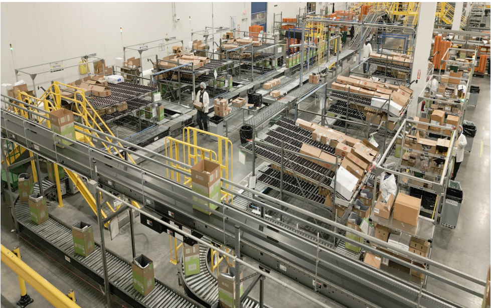
Swisslog conveyor system for light goods.
